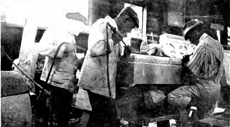
AT WORK ON THE ABBEY MEMORIAL In the yard of the Edwin Shuttleworth Co., Long Island City, N. Y.
